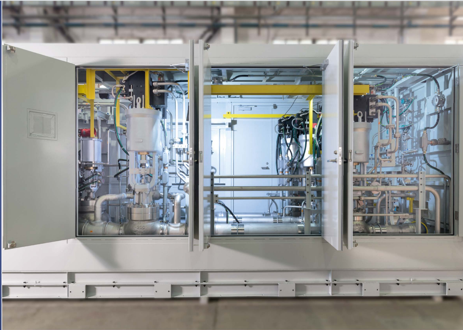
MITSUBISHI POWER M701 F4 FUEL GAS SKID
