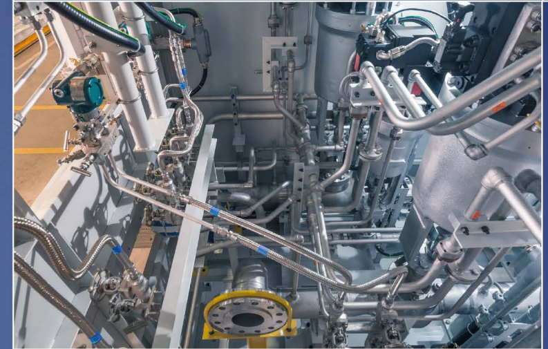
MITSUBISHI POWER M701 F4 FUEL GAS SKID
