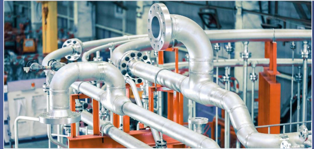
MITSUBISHI POWER AMERICA M501J JIG
