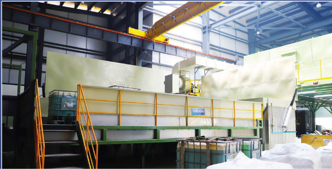
AUXILIARY EQUIPMENT STAINLESS STEEL PRE-TREATMENT AREA DIMENSIONS: 6.8*2.3*2.0m
