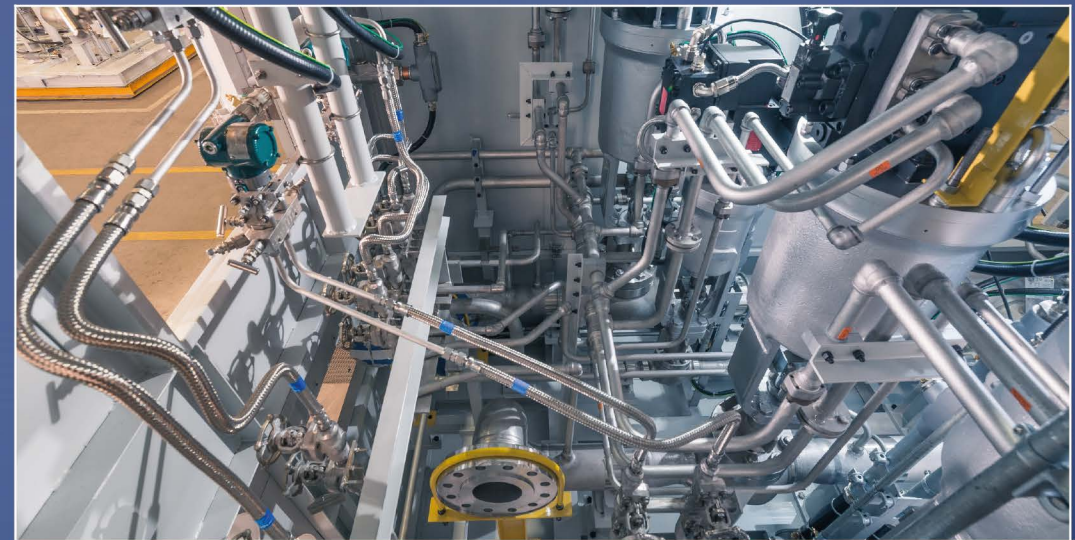
MITSUBISHI POWER M701 F4 FUEL GAS SKID
