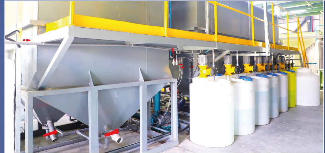
WASTE WATER TREATMENT SYSTEM CAPACITY: 2 ton/hour
