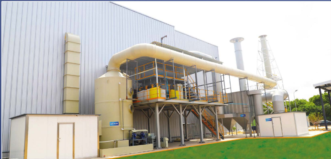
ACID MIST PURIFICATION SYSTEM CAPACITY: 40,000 m 3 /hour
