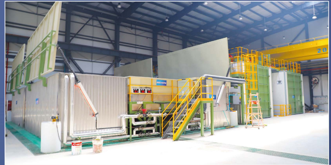
AUXILIARY EQUIPMENT CARBON STEEL PRE-TREATMENT AREA DIMENSIONS: 6.8*2.3*2.0m
