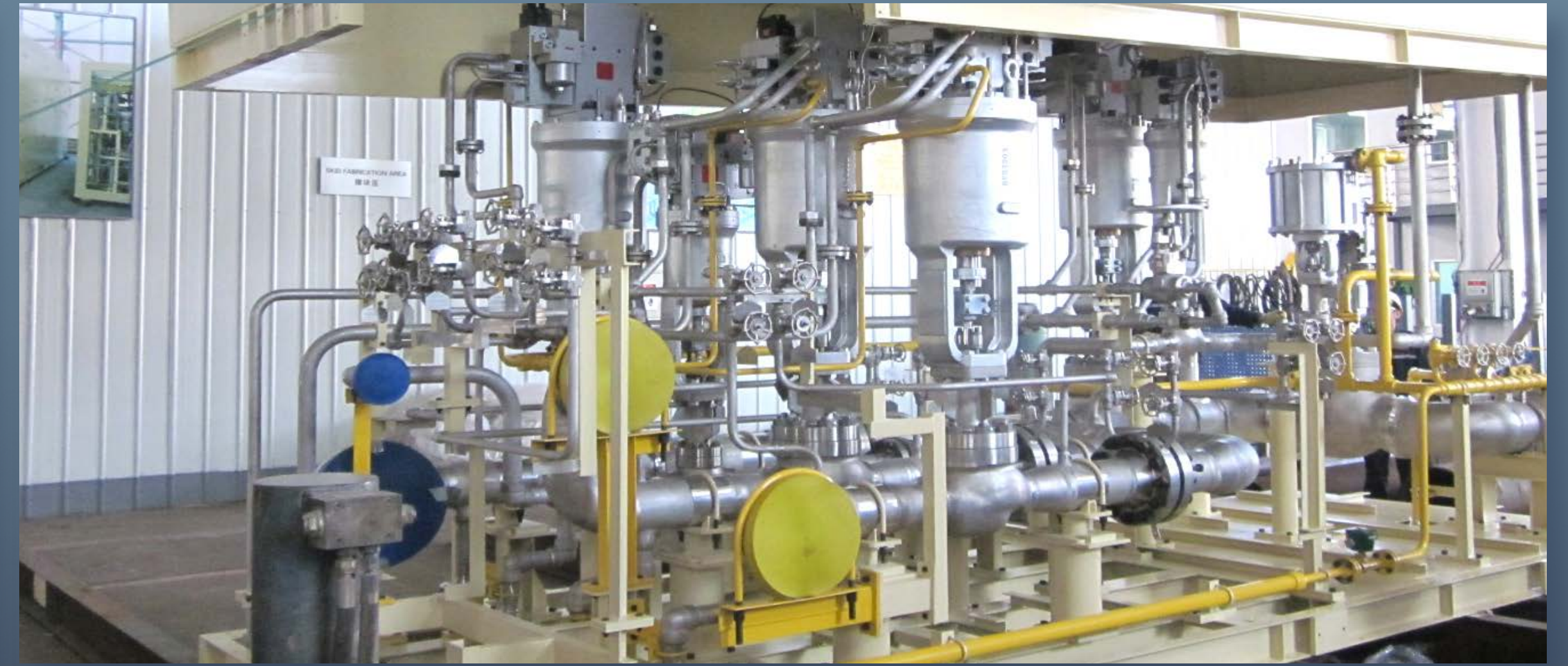
MITSUBISHI POWER FUEL GAS SKID
