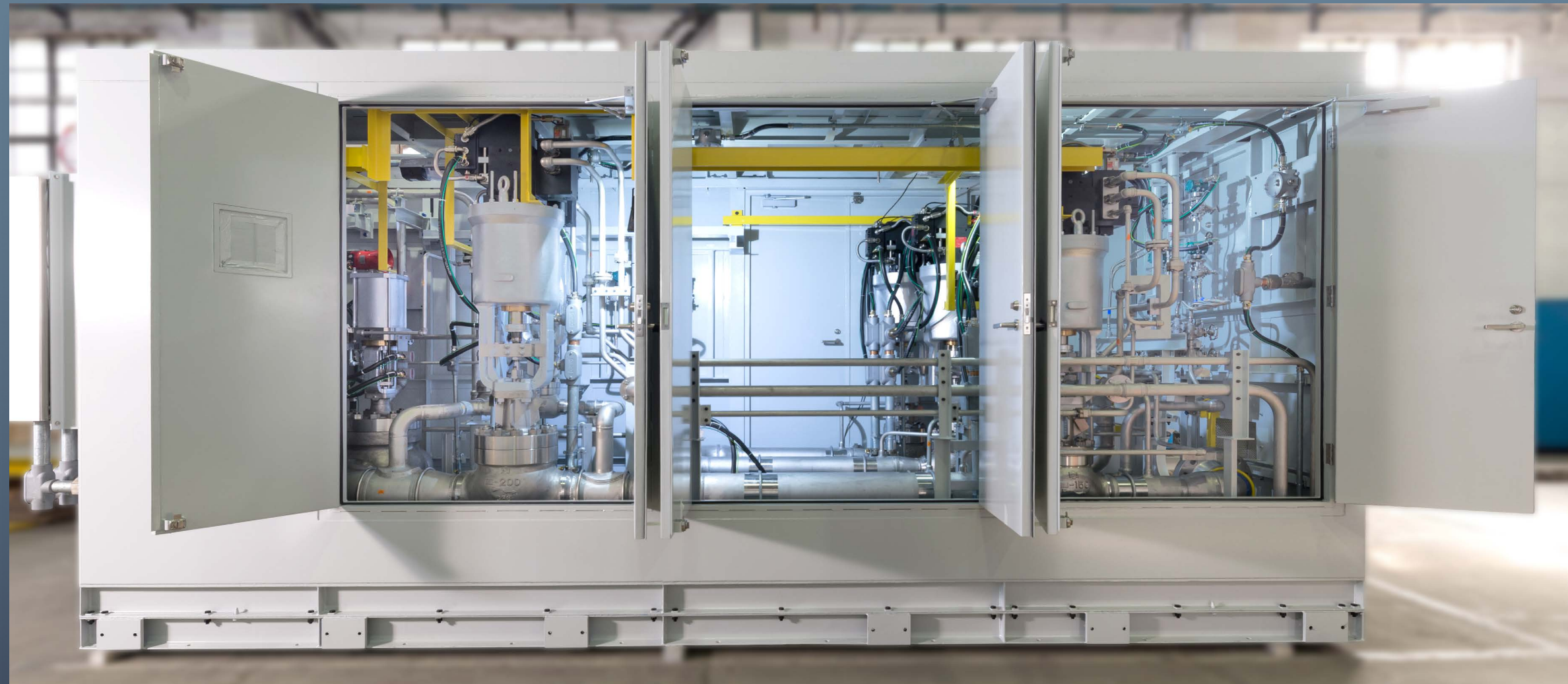
MITSUBISHI POWER M701 F4 FUEL GAS SKID
