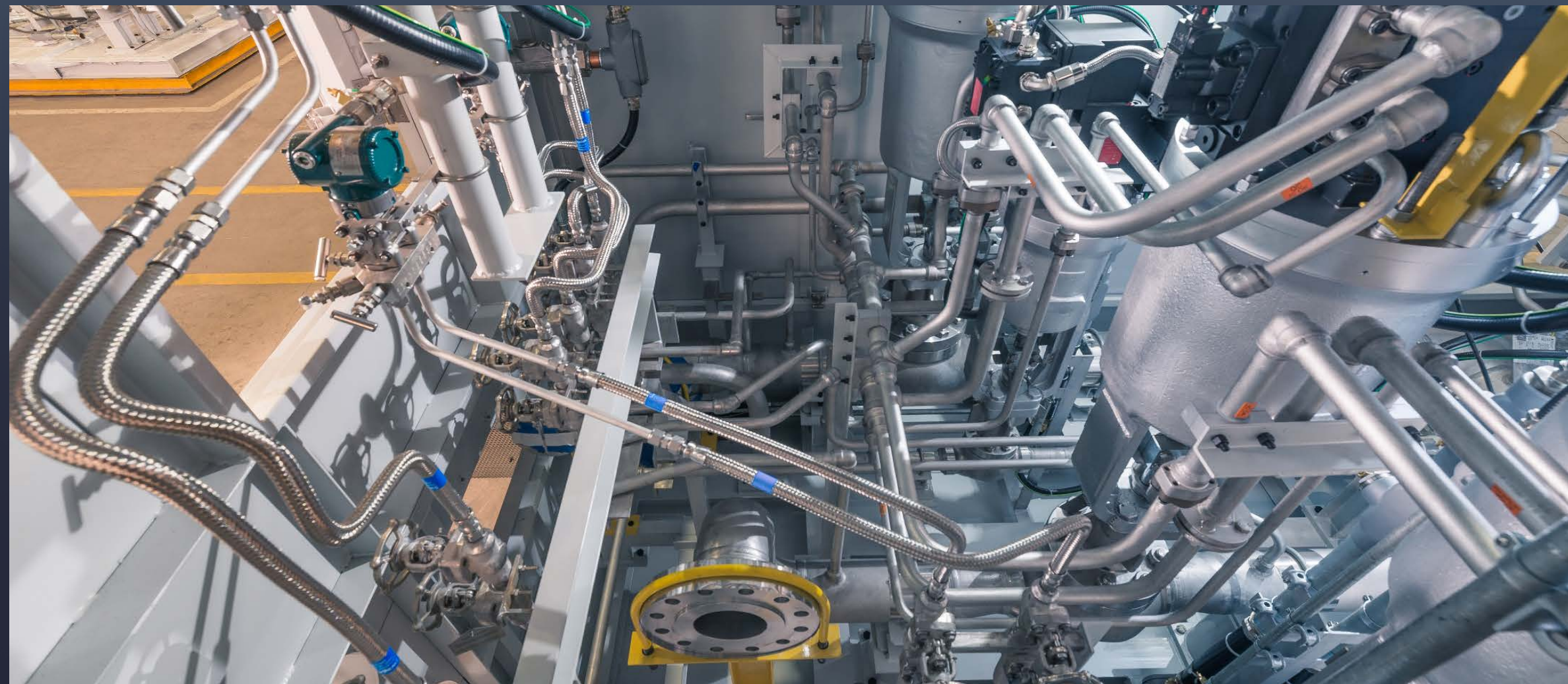
MITSUBISHI POWER M701 F4 FUEL GAS SKID
