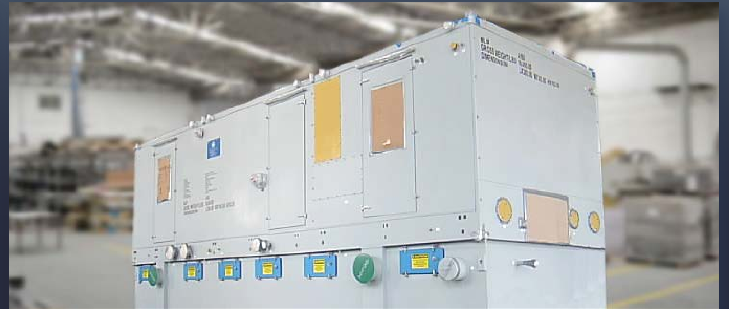
GENERAL ELECTRIC A160 SKID
